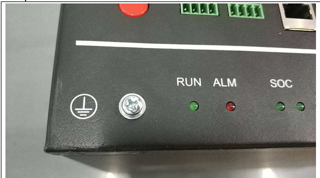
General view of Grounding terminal
